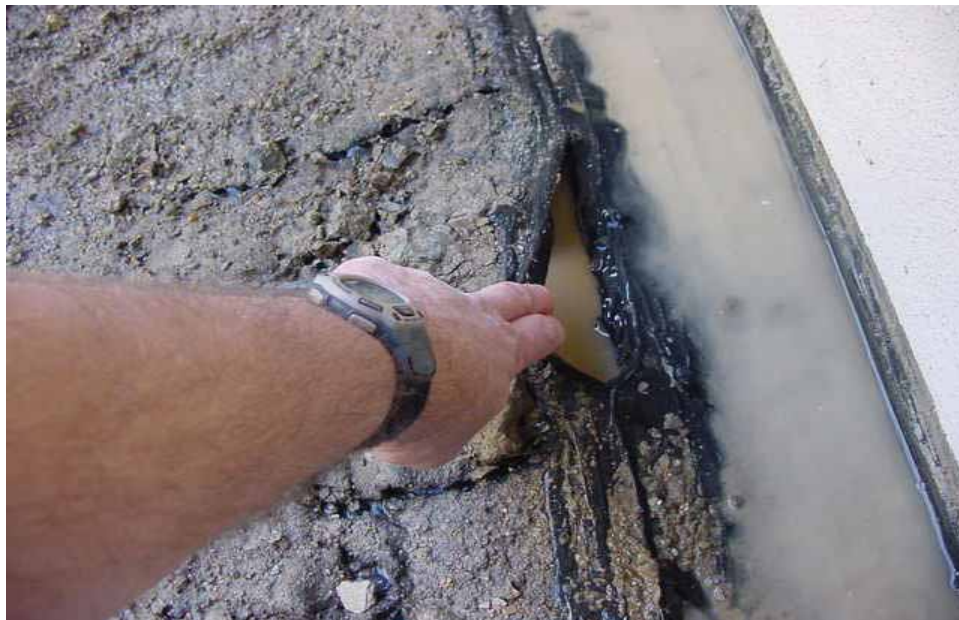
Delaminated Membrane at Flashing
