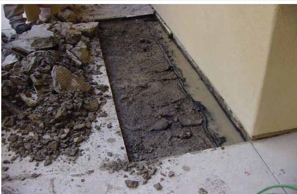
Failed Membrane Termination 33
