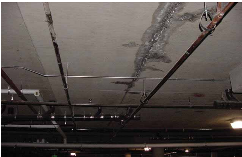
Leakage Through Podium Membrane 32
